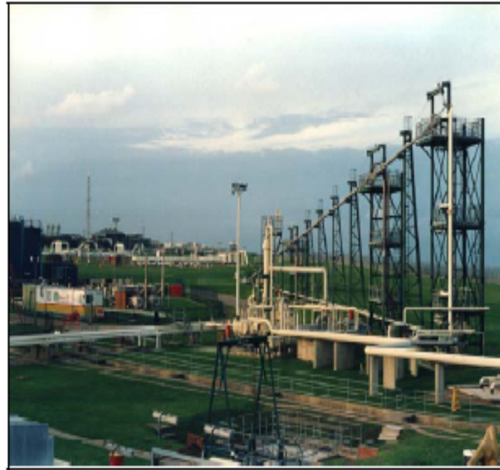
Shell test loop in Bacton (UK).
